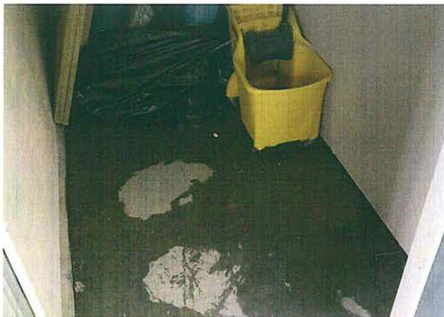
Water intrusion from neighboring unit. Discovered on a Saturday and more significant damages were avoided.
